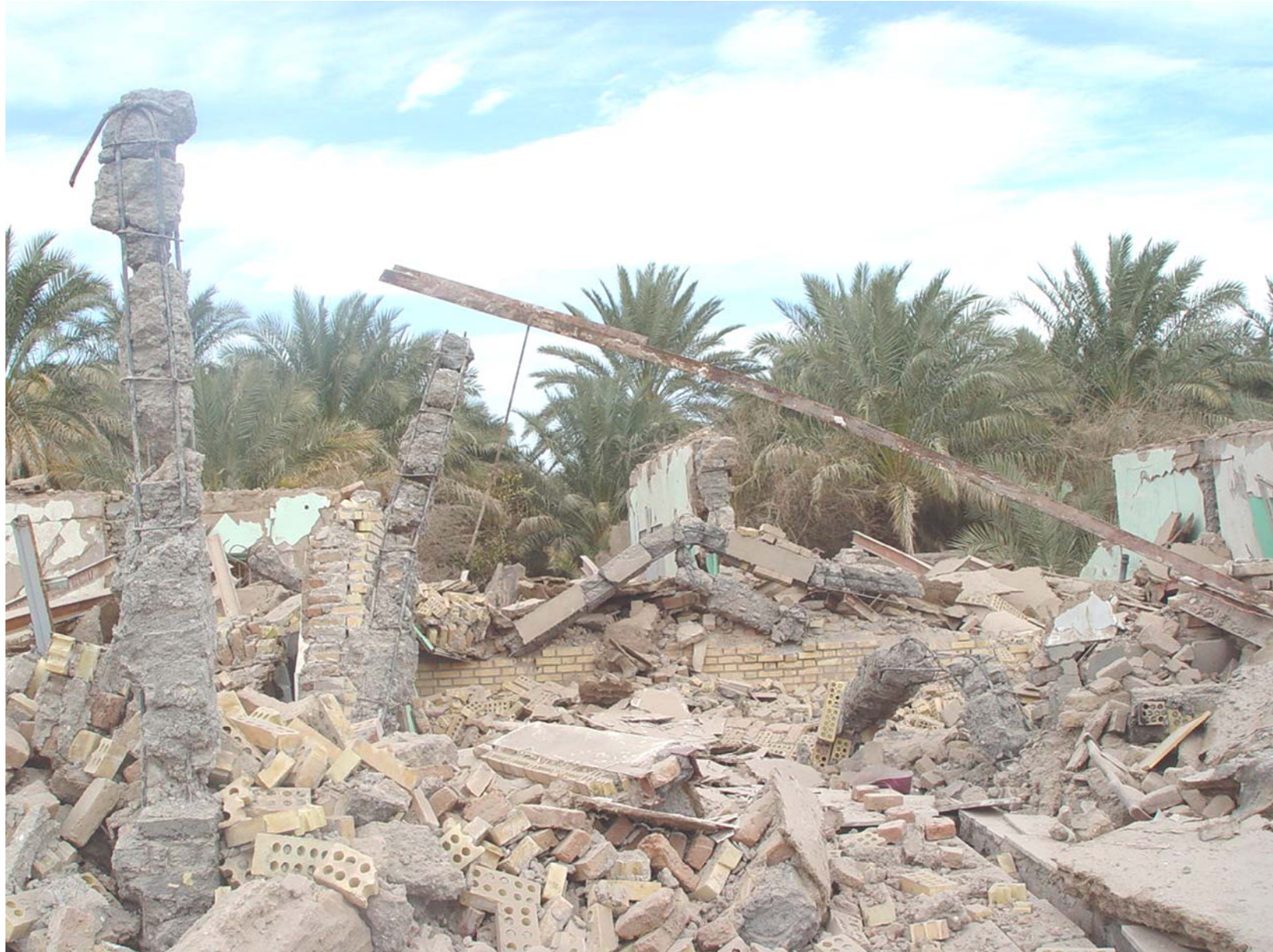
View of a confined brick masonry school that collapsed completely because of its poor construction quality and lack of proper detailing.
