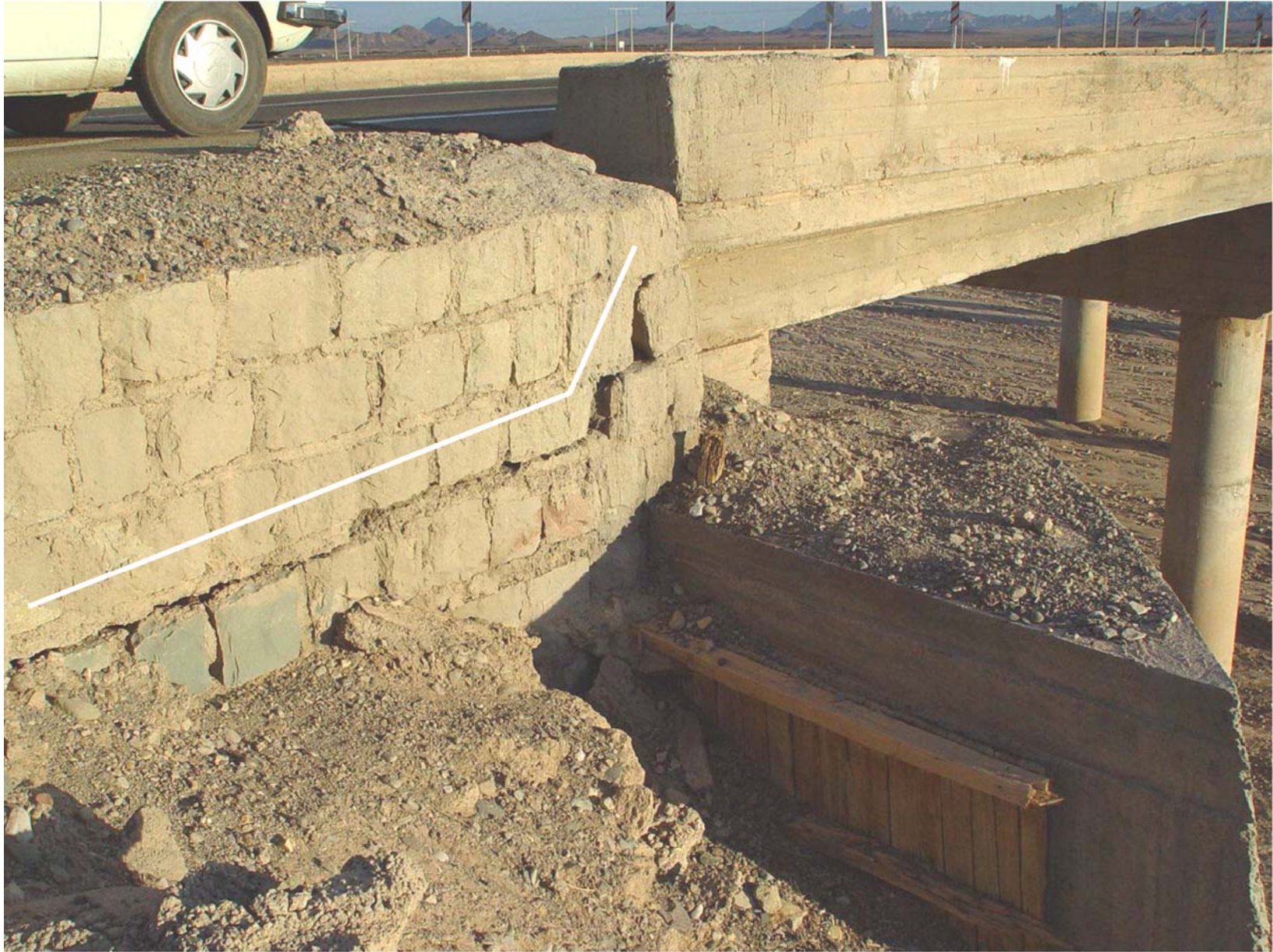
Settlement of abutment's backfill of Drazin Bridge.
