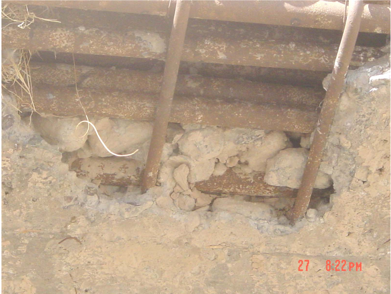
Inadequate concrete cover of beams.
