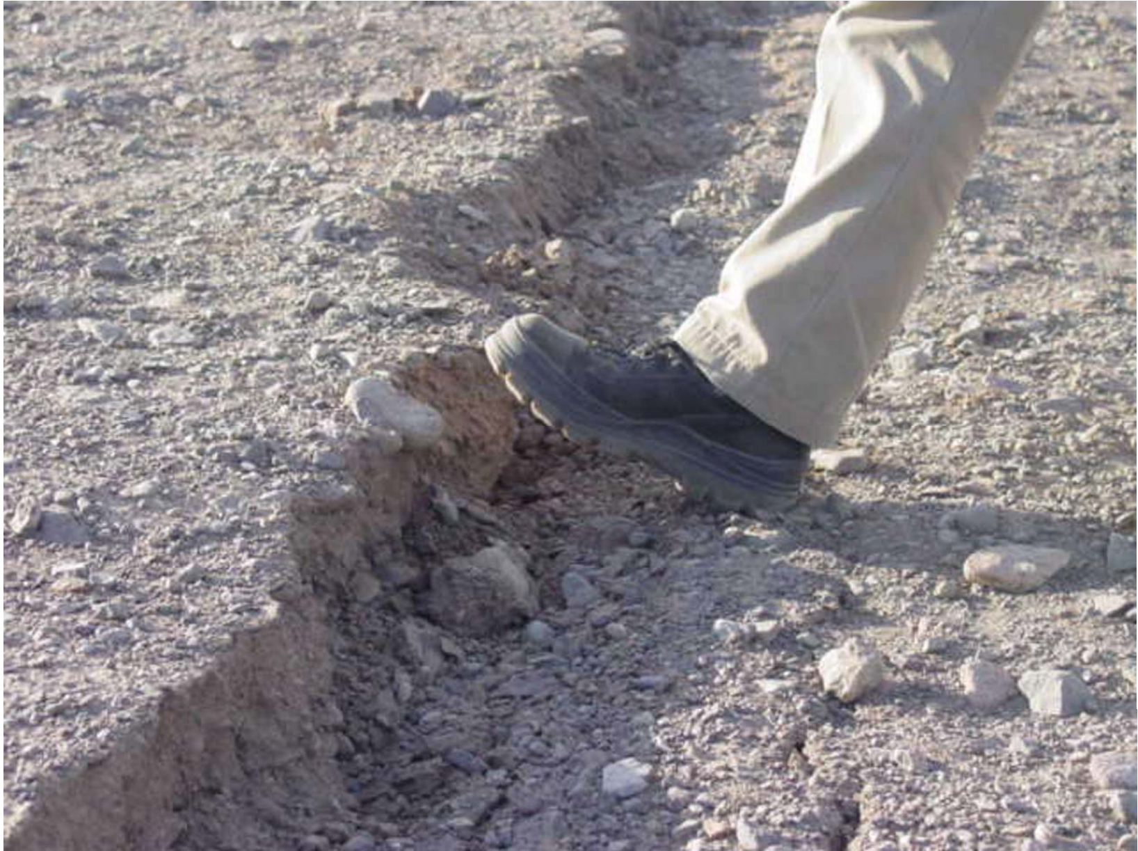
Settlement of earth fill surrounding the tank.
