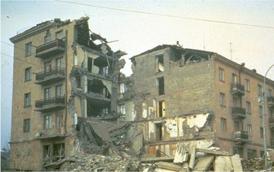
FAILURE MECHANISMS OF STONE-BEARING-WALL BUILDINGS Shows the failure of the stone bearing wall systems at the corners where the two walls meet.
