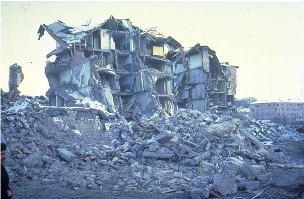
FAILURE MECHANISMS OF STONE-BEARING-WALL BUILDINGS Shows damage to a stone bearing wall building in Leninakan. The floor planks were not tied to the supporting bearing walls.
