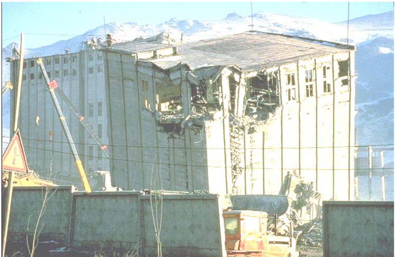
One of the collapsed cast-in-place and probably precast buildings of the granary. The building is at least the equivalent of a 10 to 15 story building. Collapse occurred in the third floor of the building which was a soft floor.
